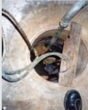
Vippor monterade i pumpgrop i pannrum.
